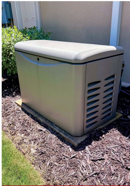
A whole-home or standby generator is wired into a home by a qualified electrician.
