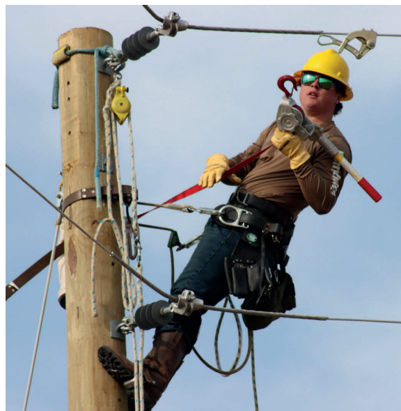
Apprentice lineman Thomas Hansen demonstrates his skills in the vertical line transfer test.
